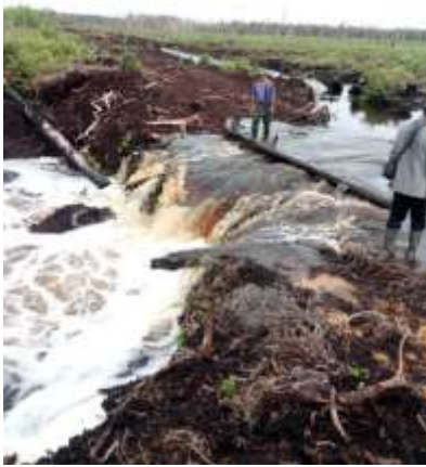
Before Repairment (photo taken 28/11/19)
